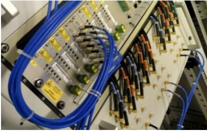
Some of the equipment that feeds the system in The Shard
